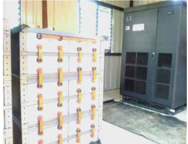
VRLA Battery Bank
